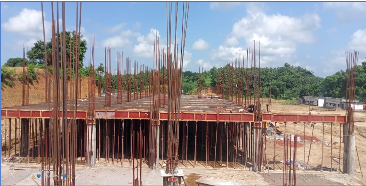
DM Building south Tripura, Agartala. Four storied administrative building. RCC frame structure, finishing, MEP Etc. Approximate area 80000 square feet. Work in progress.
