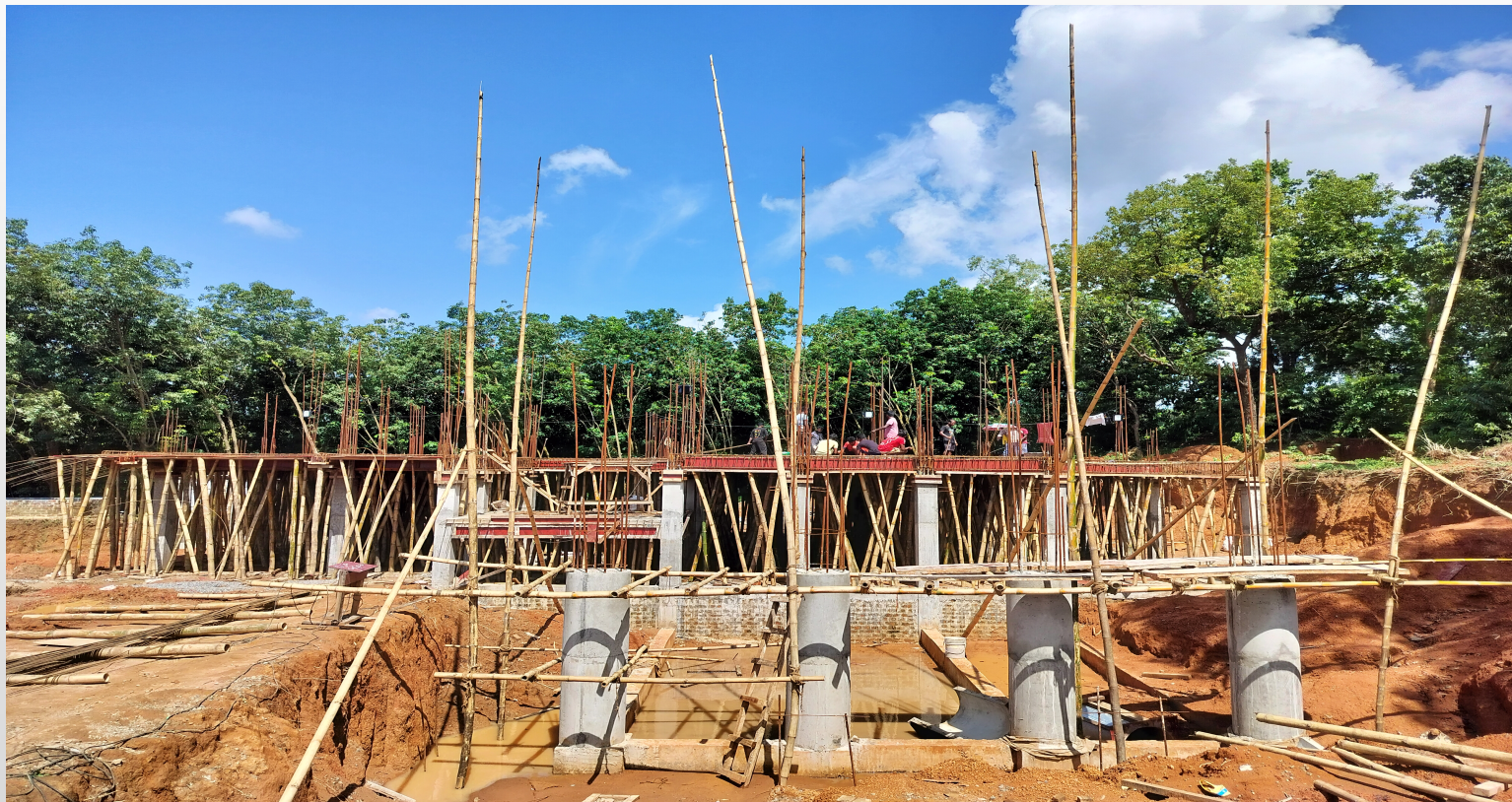
DM Banglow south Tripura, Agartala. G+1 RCC frame structure building with all finishing and MEP work. Work in progress.
